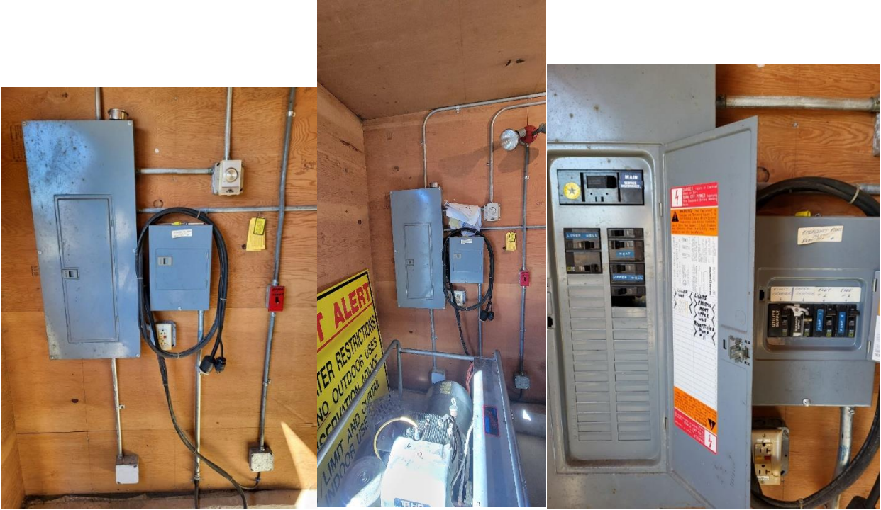
Existing panel and manual transfer switch
